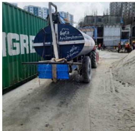
Regular road cleaning and dust prevention methods are implemented at the FDC work site.
